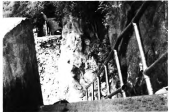
Photo 4. A portion of the collapsed staircase with prominent gap along the interface.
