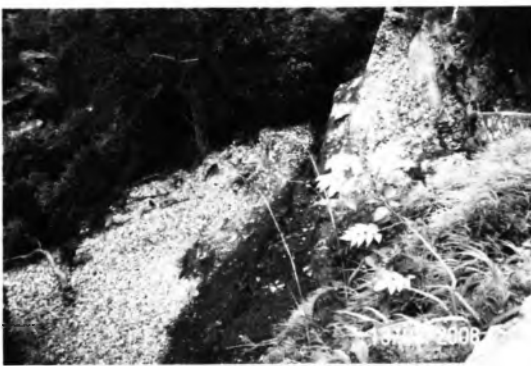
Photo 3. The collapsed staircase structure and its debris.
